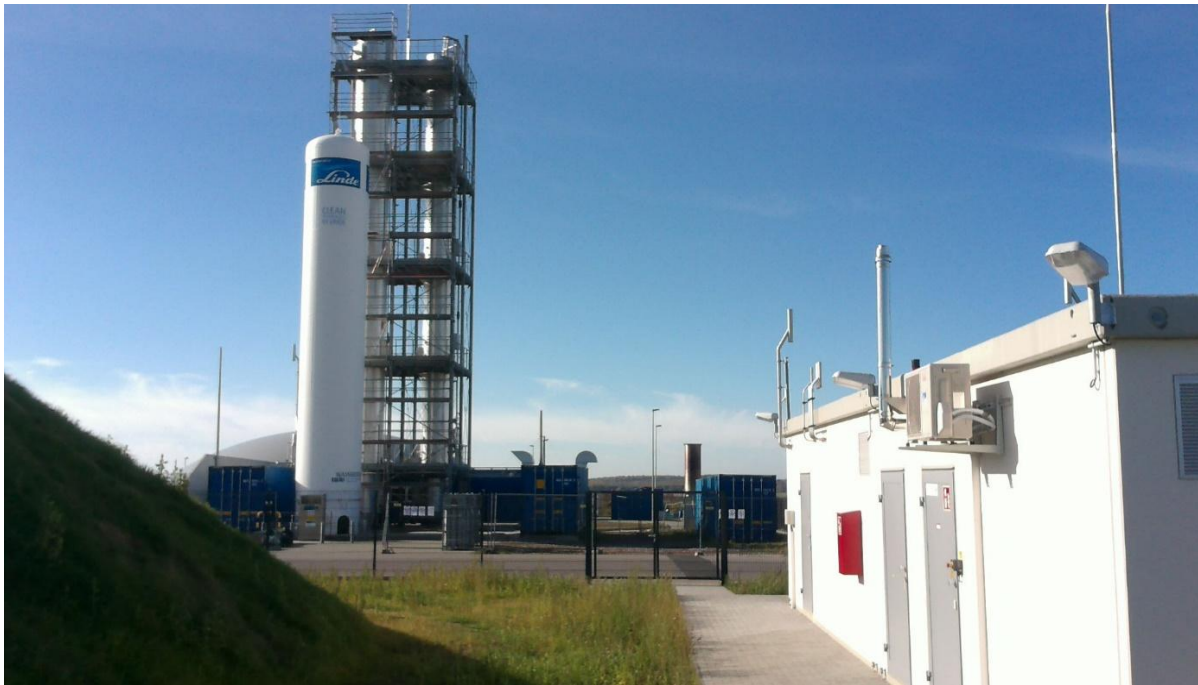
PFI biogas conditioning unit (back left) and the biogas feed-in unit of the Pirmasens municipal utility company (front right) at Pirmasens-Winzeln Energy Park
