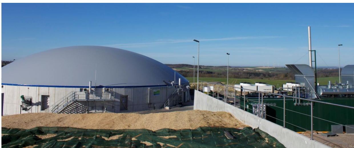
Fig. 3: Plant (container) and CHP
