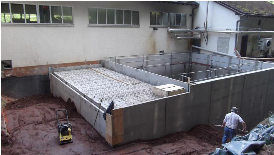
Concrete basin for the high-performance digester and MAP crystallisation unit behind the machine hall
