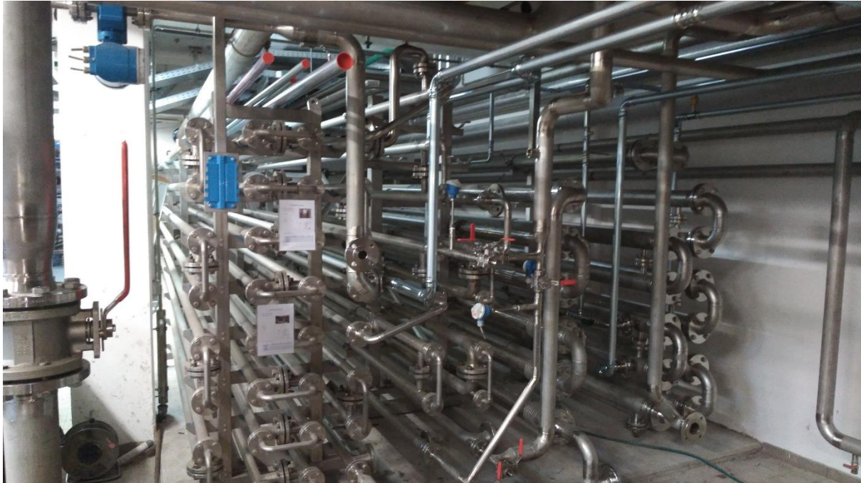
Fig. 3: Heat exchanger of the high- pressure thermal hydrolysis unit in the basement of the machine hall
