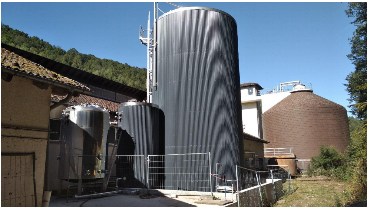
Fig. 2: Rear view of the machine hall with the new high-performance digestion system (centre), additional vessels for phosphorus recovery (left) as well as the existing digestion tower (right)
